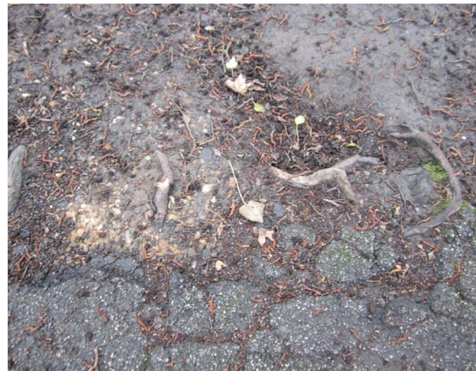
Damage to macadam due to tree roots
