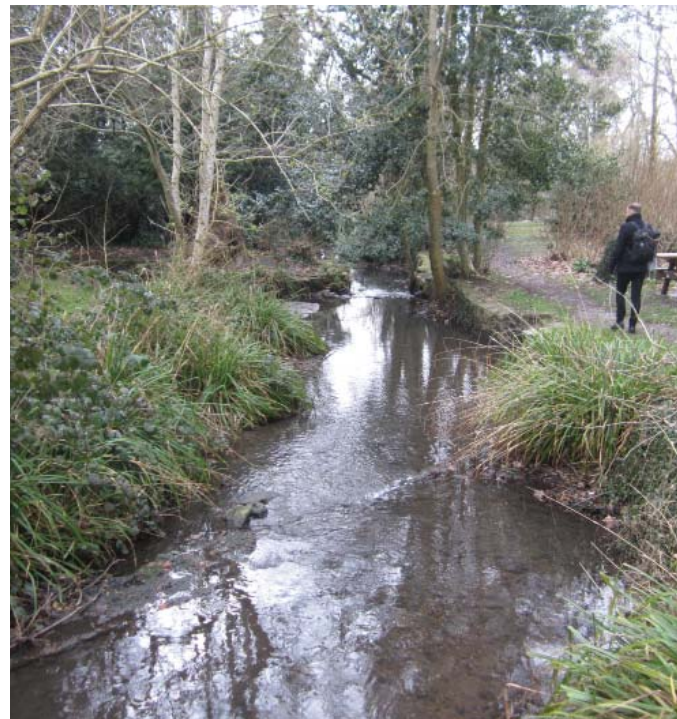
Vegetation beginning to break up wall structures
