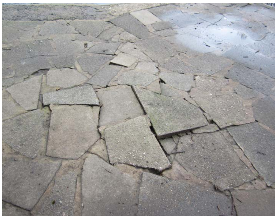
Hazardous crazy paving in need of repair
