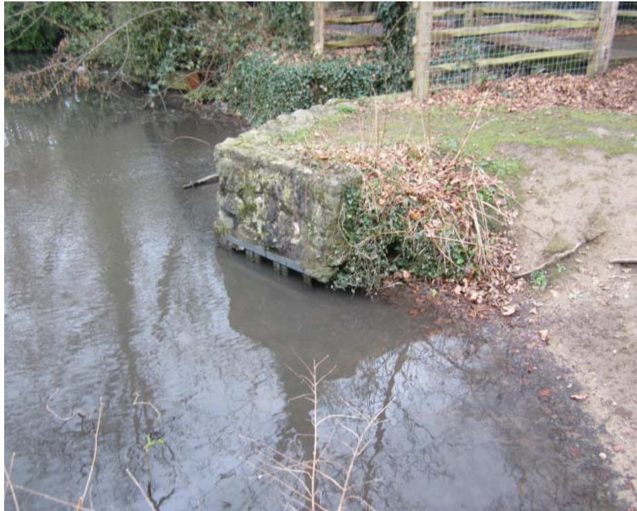
Eroded lake banks in central lake
