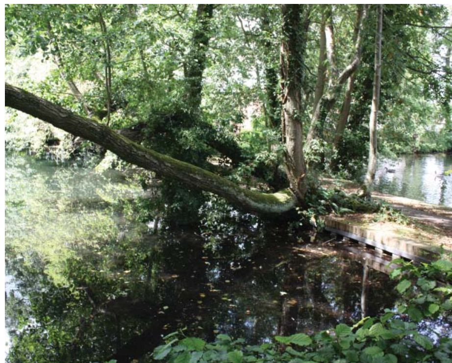
Naturalised trees damaging edges
